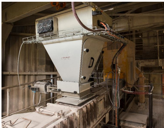
SpectraFlow Analyzer on an airslide in a cement plant
