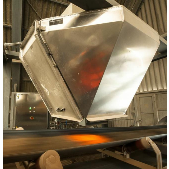
Analyzer in a cement plant
